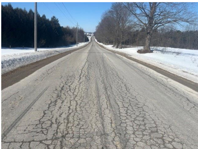
Large alligator cracking
