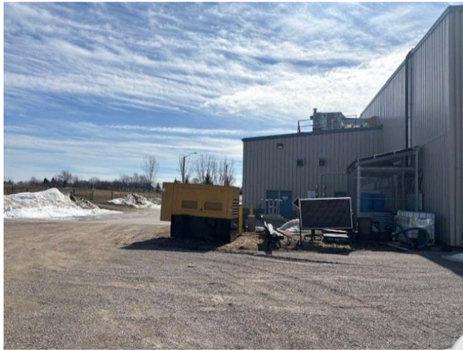
Generator to be installed.
